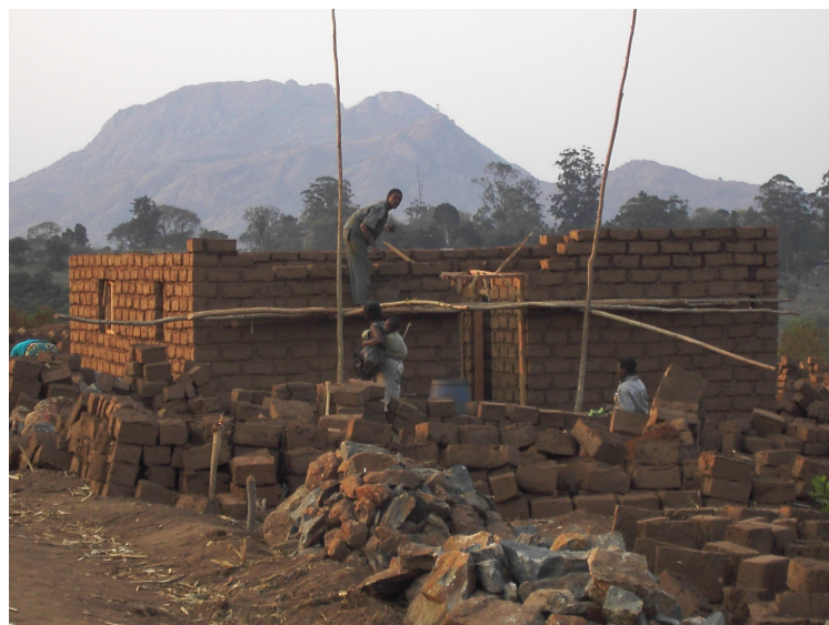
Low-cost housing production in Kanjedza, Blantyre by Malawi Homeless People's Federation © R. Precht
