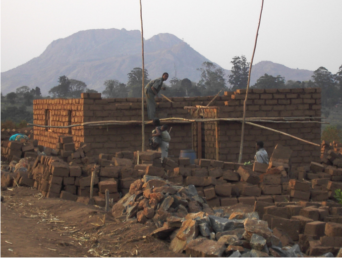
Low-cost housing production in Kanjedza, Blantyre by Malawi Homeless People's Federation © R. Precht
